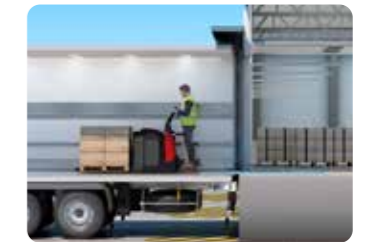
3. Ongoing loading operations, no safety.
